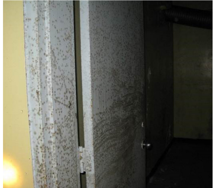
Mold growth in poorly ventilated space
